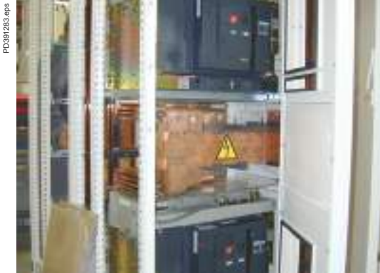
Source changeover system in the same cubicle.
