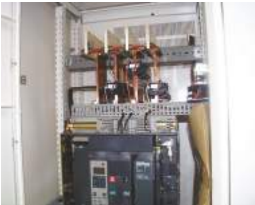
CT on vertical busbars.
